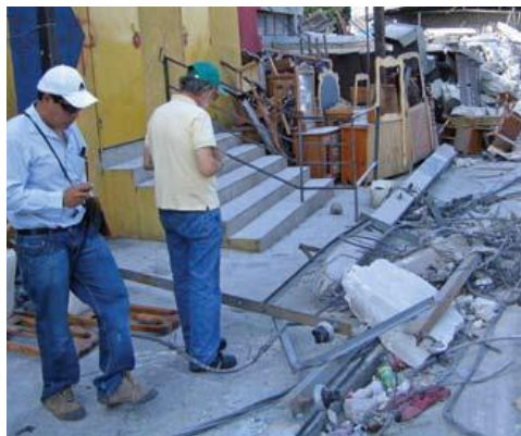
NRECA volunteers survey a tangled mess of damaged power lines in Port au Prince, in the days following Haiti's January 12 earthquake.
