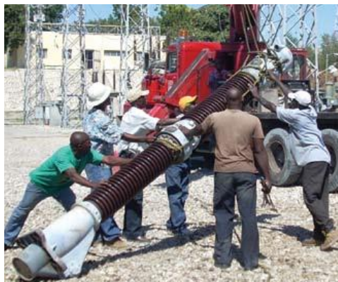
A crew from EdH, Haiti's main electrical utility, work to repair a substation in the aftermath of the January 12 earthquake.
